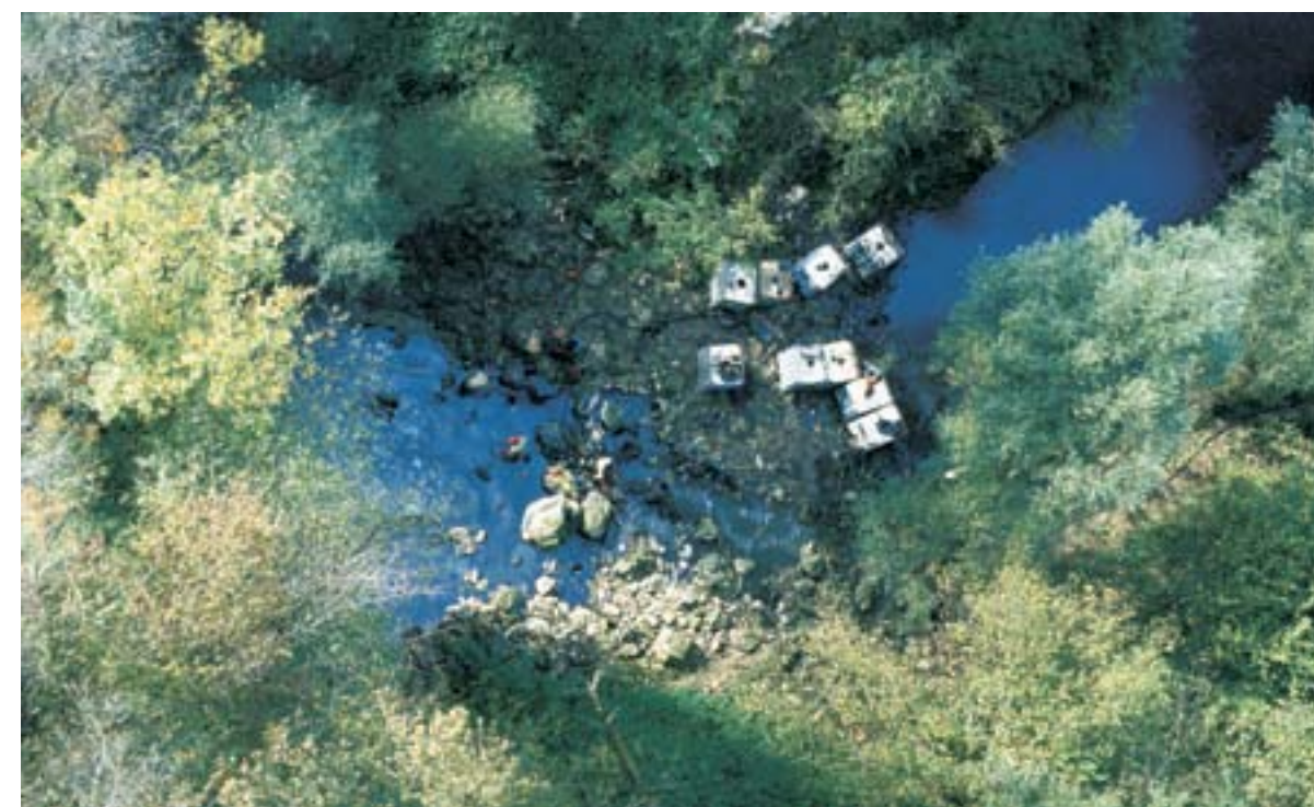
Fig. 3: Cleaning fuel oil from the bed of the Pazinčica
