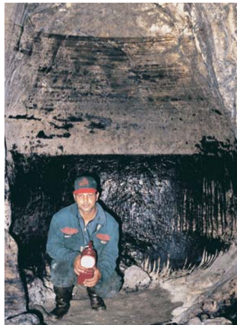
Fig. 5: Traces of previous, unrecorded accidents.
